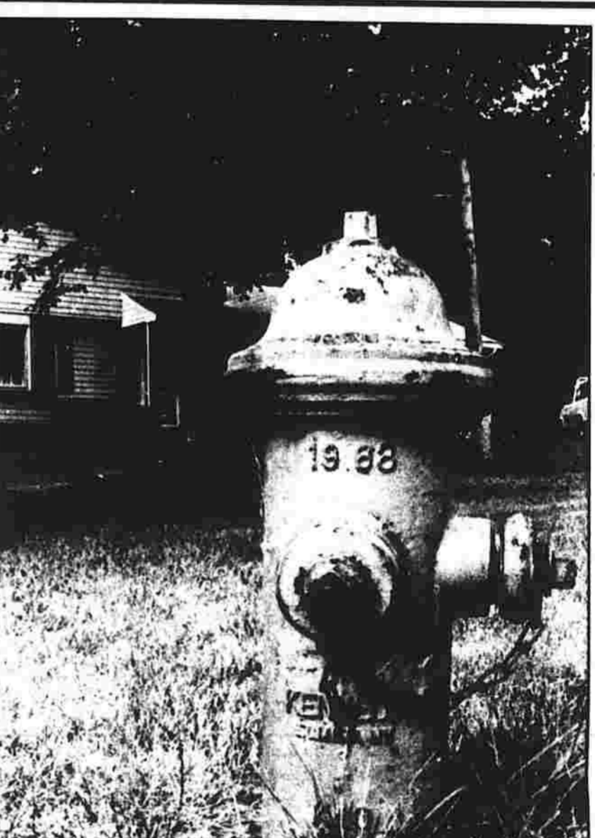
This fire hydrant, as well as seven others in the Redwood Farms subdivision of southwest Manchester, has never been operable for fire protection purposes.
