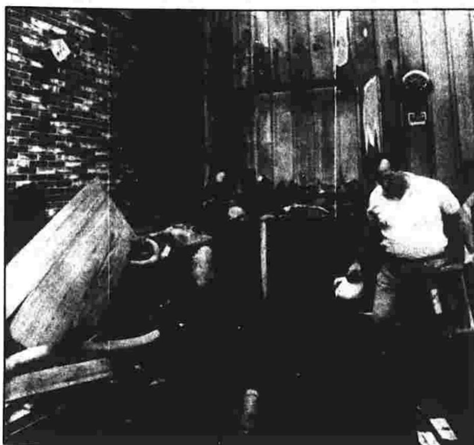
An employee of Arthur Industries checks on the damage caused by a gas explosion Monday afternoon at the South Main Street plant in Plymouth. The explosion blew flames into the air, injuring two workers of Connecticut Light & Power, and shattered windows in a nearby building.
